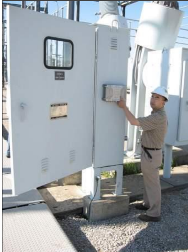
External, on a Circuit Breaker
