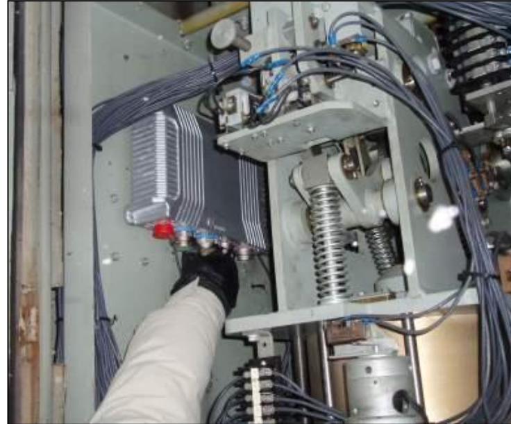
Internal, old oil-type Circuit Breaker
